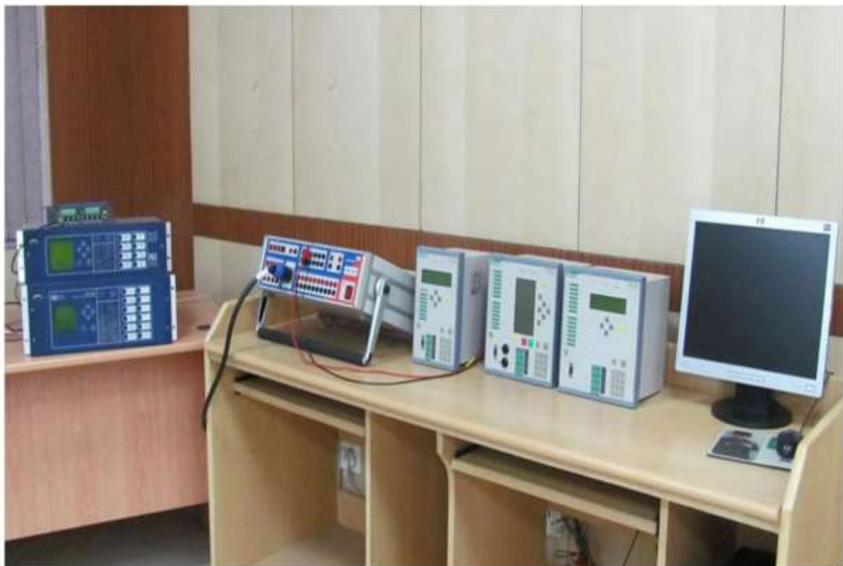
Fig. SCADA and Smart Grid RTDS Laboratory Equipments
